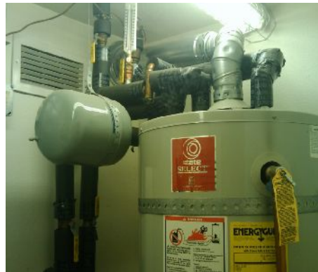
Hot water demand in facility is low. This heater may not be necessary and costs a minimum of $300/year to operate.
