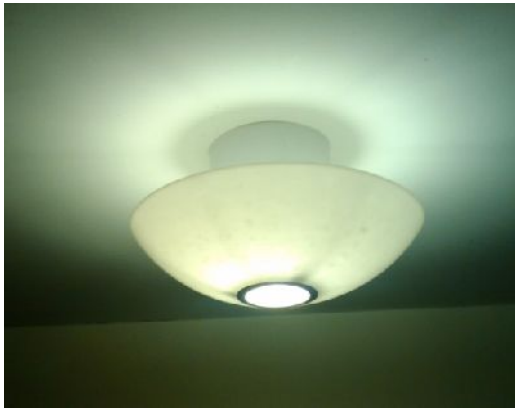
Pendant light fixture with CFL lamp.
